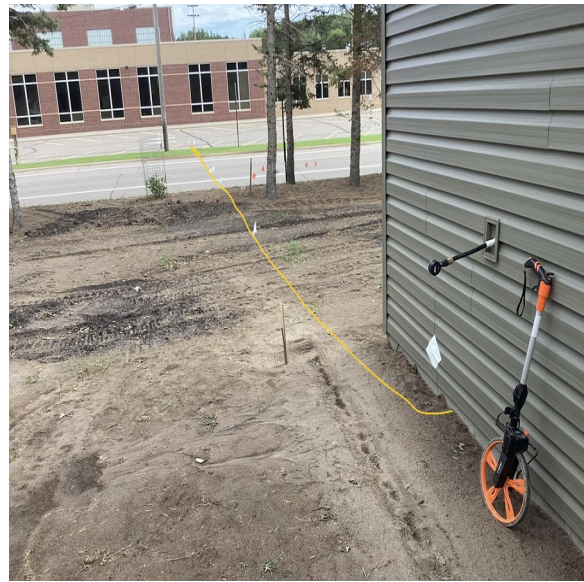
Gas meter location
